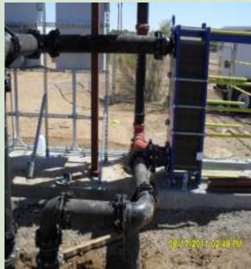
Photo of the Church HVAC system under construction, including influent and effluent conveyance piping connecting to the plate and frame heat exchanger.
