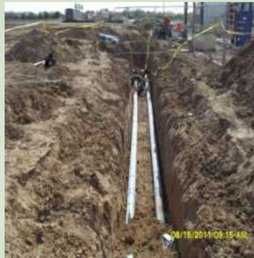
Photo of influent and effluent underground conveyance piping from the treated effluent primary line to the Church HVAC system, providing treated groundwater for use as non-contact cooling water.
